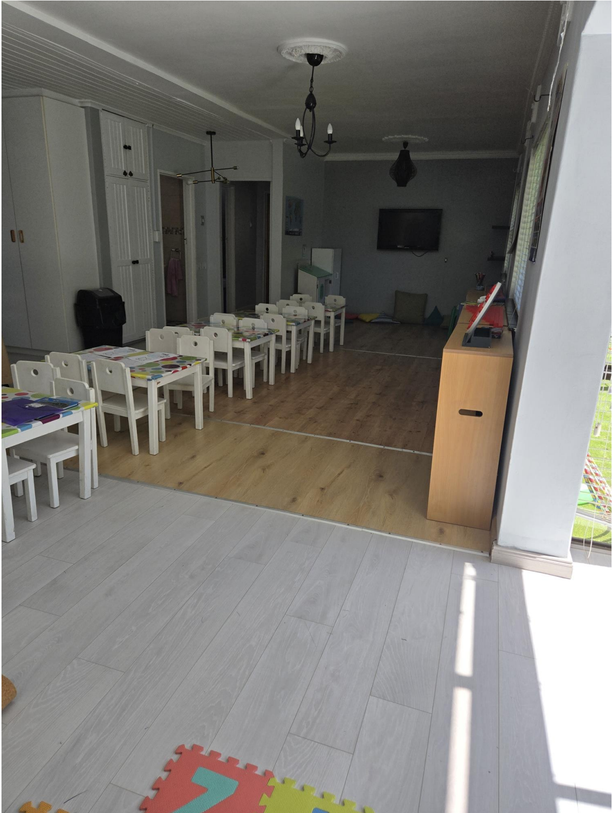
Fig. 3 No. 4 Fiona Crescent – Early Learning Centre - Large Classroom 2 (following the demolition of the internal walls)
